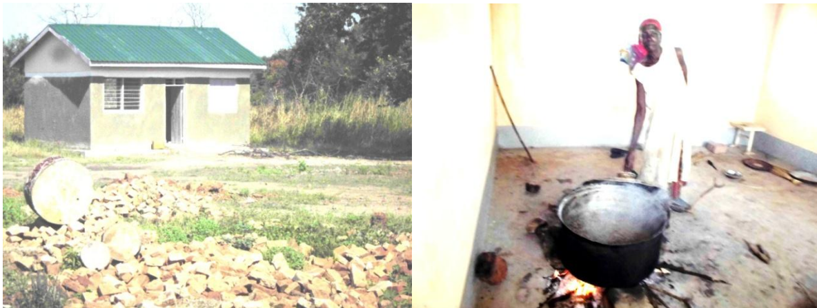
Figure 18: Kitchen/Storage (lacking chimney) and Cooking stove on the floor in Warahel Primary school. Photo: J. Makongo.
